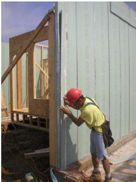
Worker using gypsum liner board to ensure steel framing end cap stays in place.
